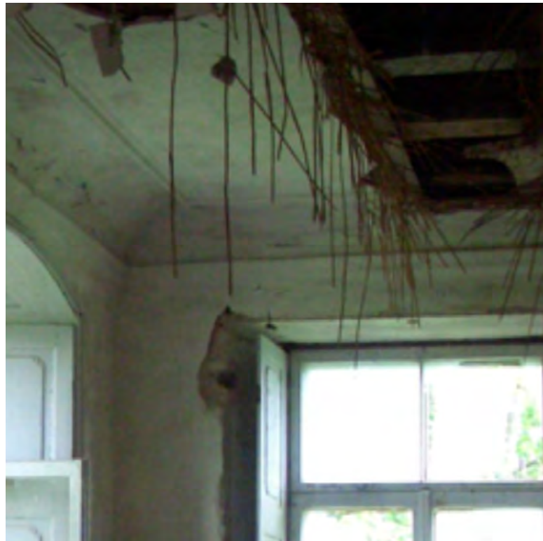
Figure 3.41. In some of the rooms at Seidla only the paintwork is damaged otherwise the cornice is in good condition.
