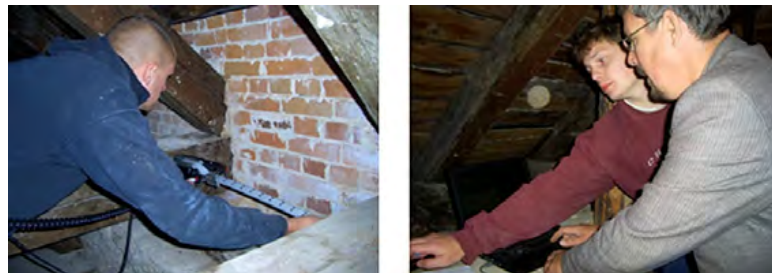
Figures 3.14. One student is drilling into a roof truss while the other is learning to interpret the transmitted information on the computer. Prof. Kalle Pilt, lecturer at Estonian University of life Sciences, (far right) is explaining the curves on his computer screen.
