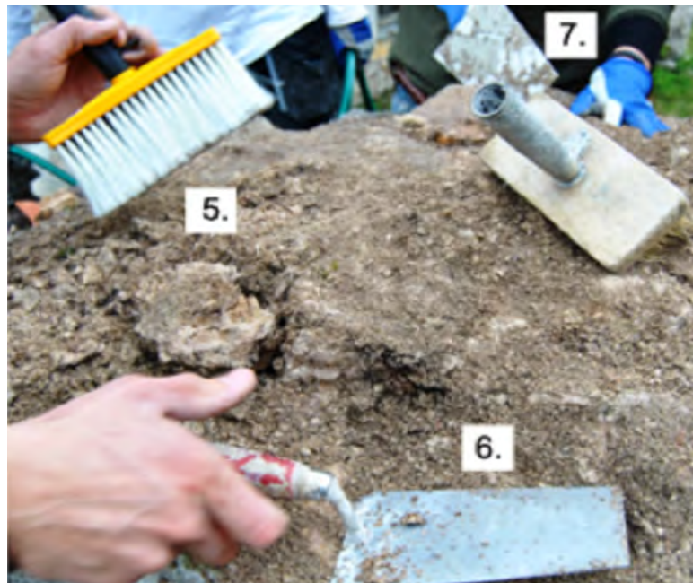
Figure 2.11. More tools: brushes (5)—used to wipe off sand and also to even out mortar on the sides of the posts; trowels (6)—used to apply the mortar onto the wall; waterproof gloves (7)—used when handling the mortar to prevent direct contact with lime; tape measures used for documentation.
