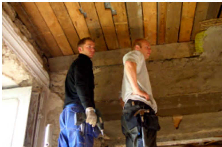
Figure 3.45. Well done! Only another few hundred meters to go... the two engineers are waiting for more instructions from the Master of Seidla, supervisor of all the work we performed.
