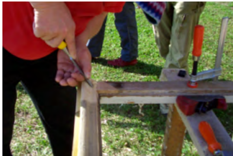
Figure 3.38. The new patch of the weather moulding is being shaped to match the old parts.
