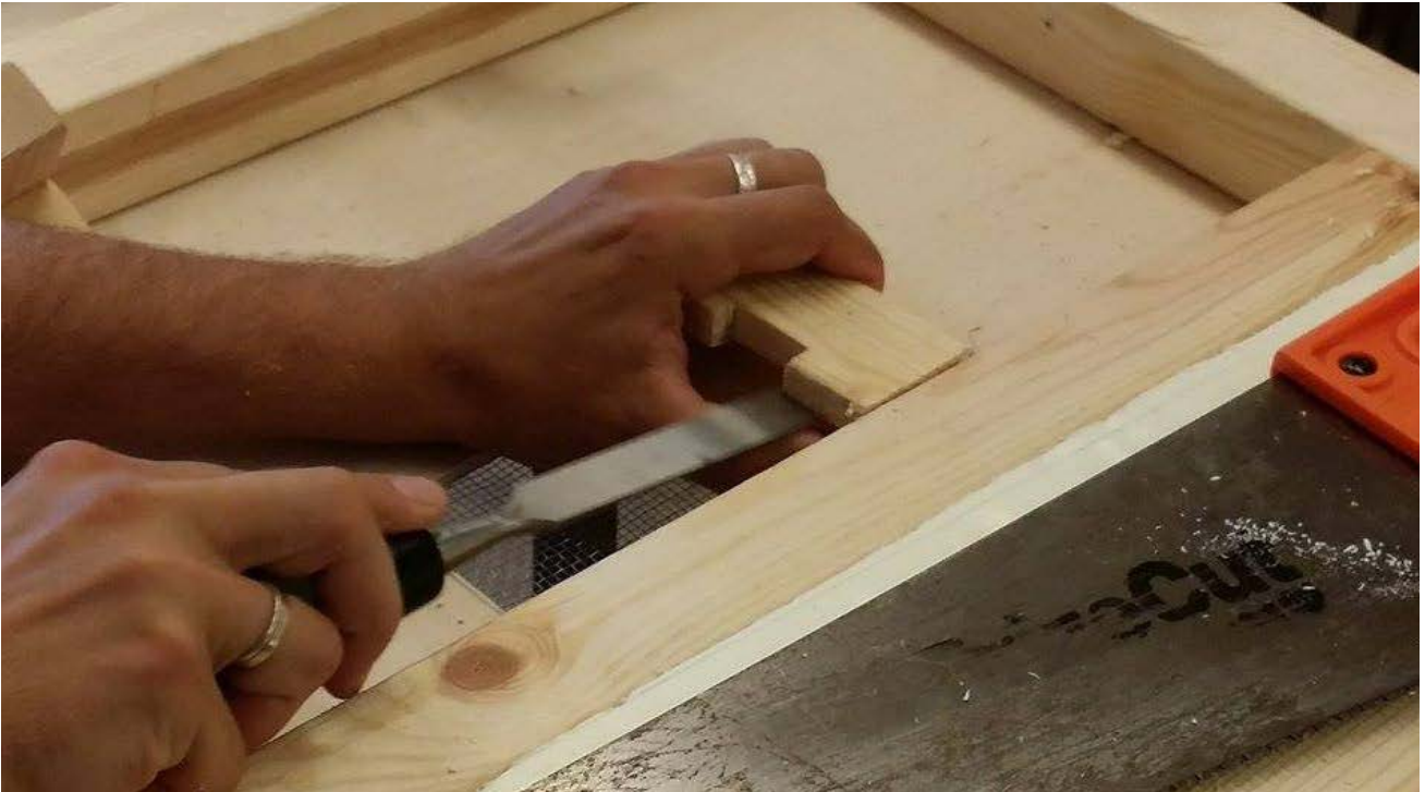
FIGURE 4.2. The air vent is being built at the bottom part of the door. Photograph by Aulden Carter.
