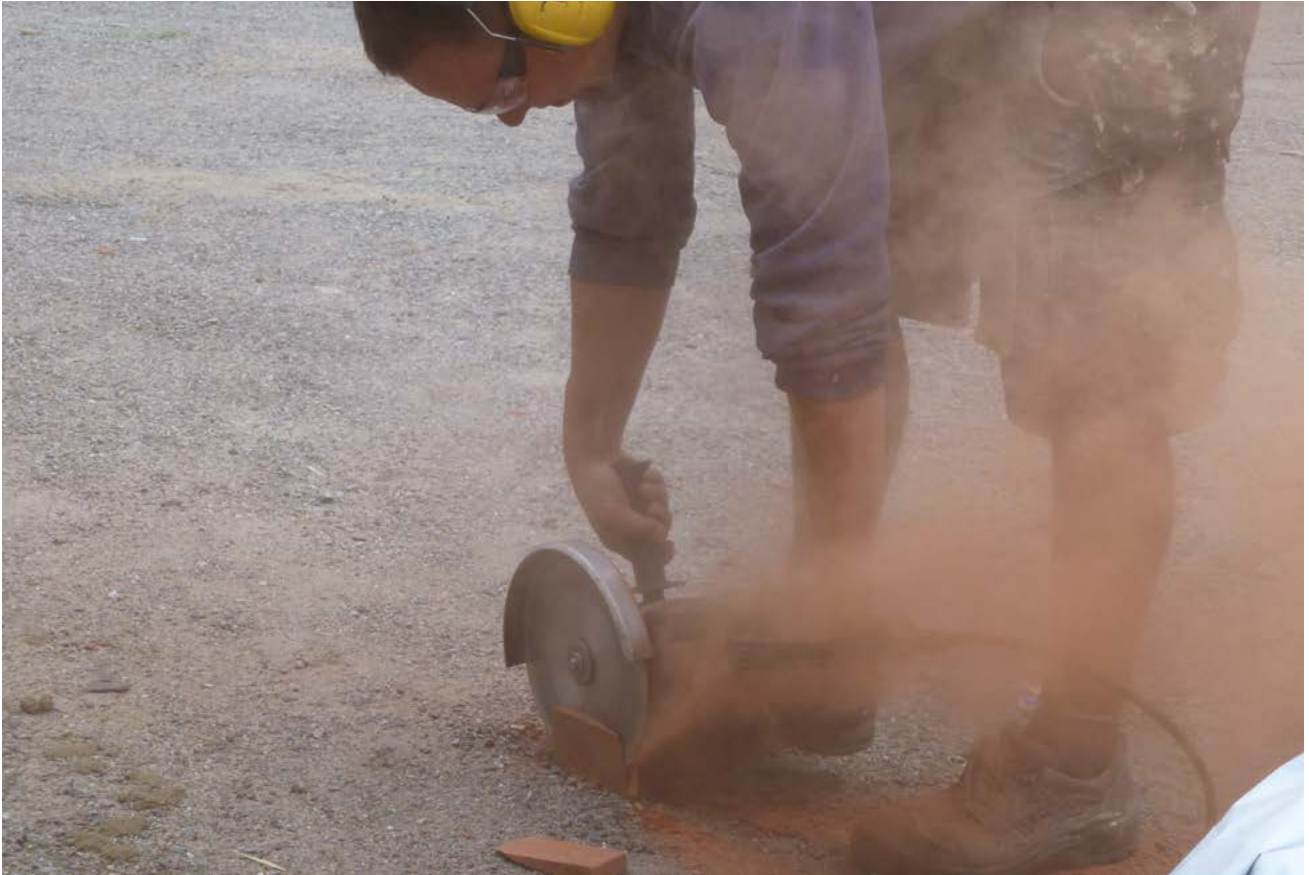
FIGURE 2.22. Cutting bricks with a circular saw is dusty and hazardous work; not a job for inexperienced people! It could be done with a brick guillotine or a mason's hammer as well but the cut would not be precise. Photograph by Kirsti Horn.
