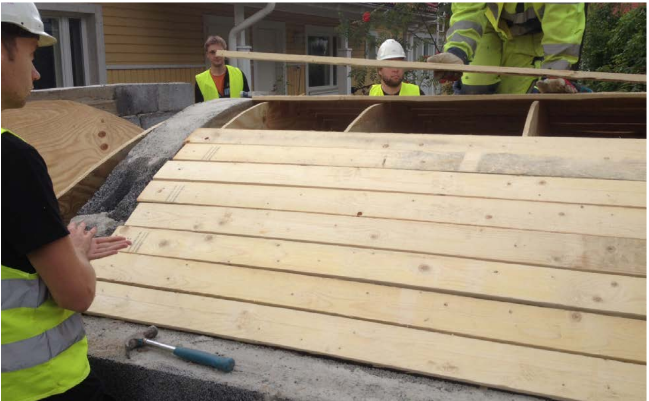
FIGURE 2.14. The centering for the storage room vault is completed by boards nailed onto the plywood sheets. Photograph by Sanna Svensson.
