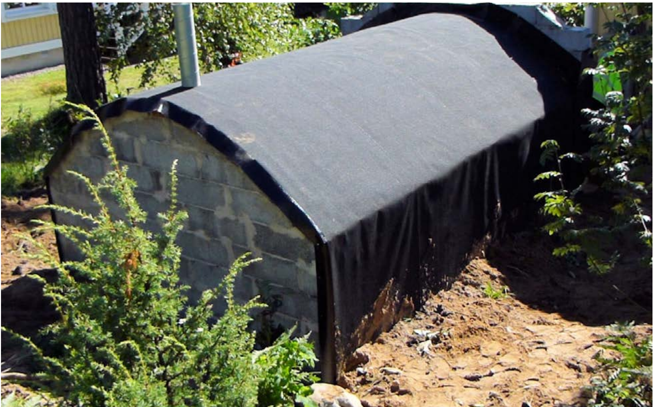
FIGURE 2.26. The finished damp proofing gives mainly protection from rain. A French drain was placed along the plinth around the whole building to lead excess water away from the masonry. Note how the felt has been bent over the joint between brick vault and concrete blocks at both ends. The back of the cellar will be hidden by sand which will allow some necessary humidity through the wall into the cellar. Photograph by Kirsti Horn.
