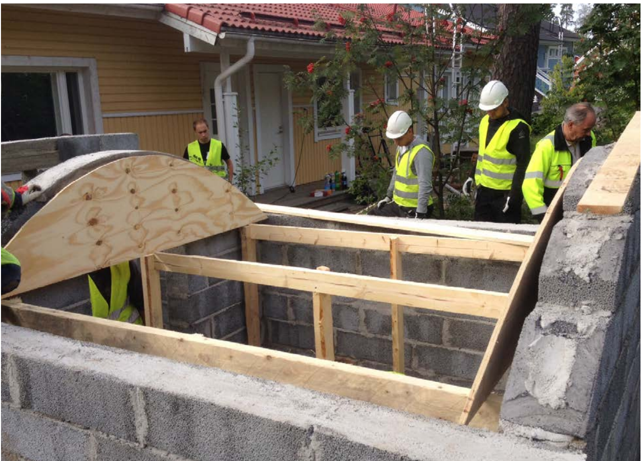
FIGURES 2.12. The centering rests on a structure of beams and posts which matches the height of the room. Photograph by Sanna Svensson.
