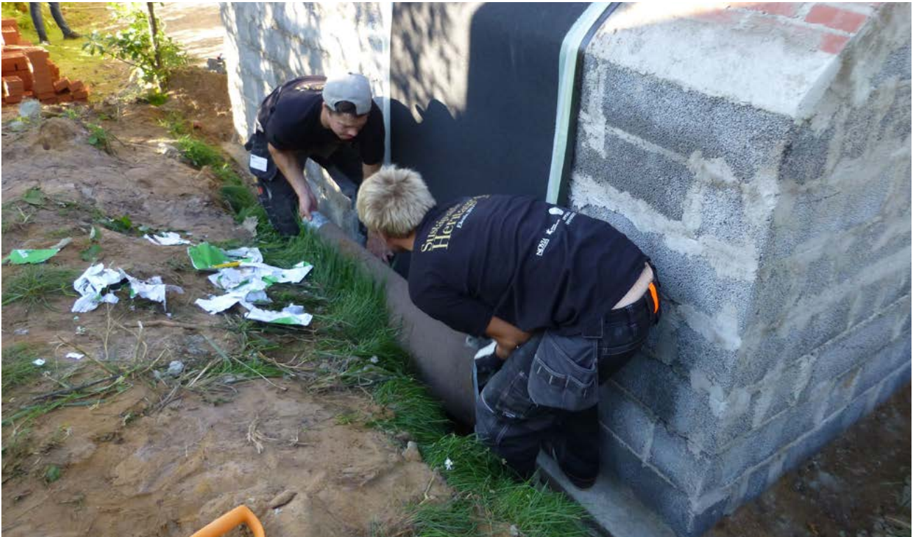
FIGURE 2.25. The felt is being measured long enough to protect vault, walls and the top of the plinth from rainwater. Photograph by Kirsti Horn.
