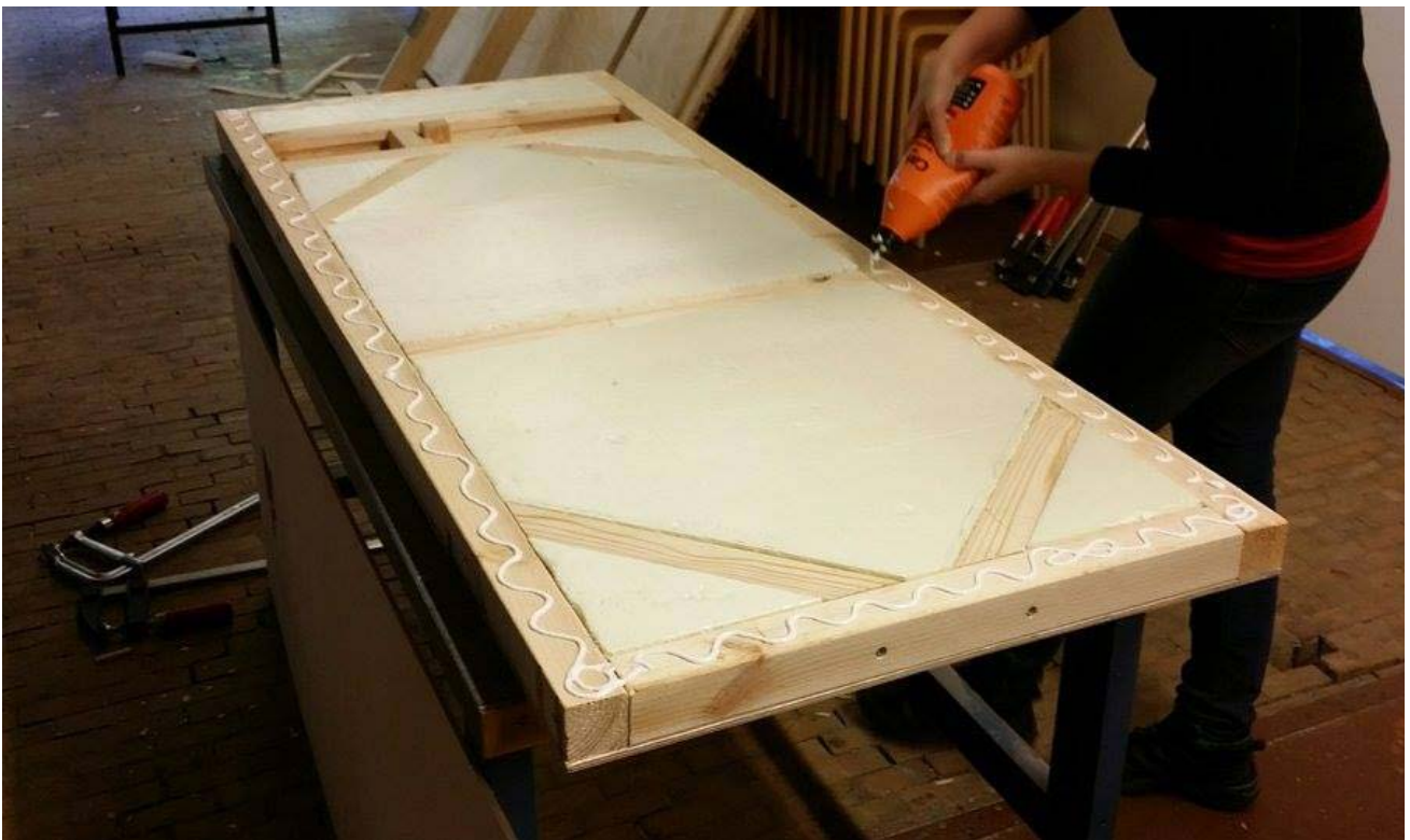
FIGURE 4.5. Polystyrene insulation in place; glue for the inner sheet of plywood is being spread onto the framework. Photograph by Aulden Carter.
