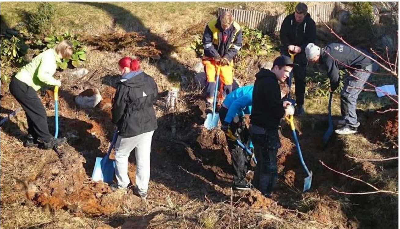
FIGURE 2.1. The sandy slope between two houses is an ideal spot for the model root cellar. Photograph by Niklas Nyman.
