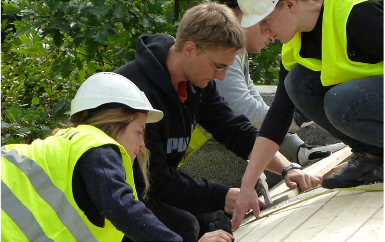
FIGURE 2.17. Positions for the brick courses are being marked on the centering. It is important that joints are uniform. Photograph by Kirsti Horn.
