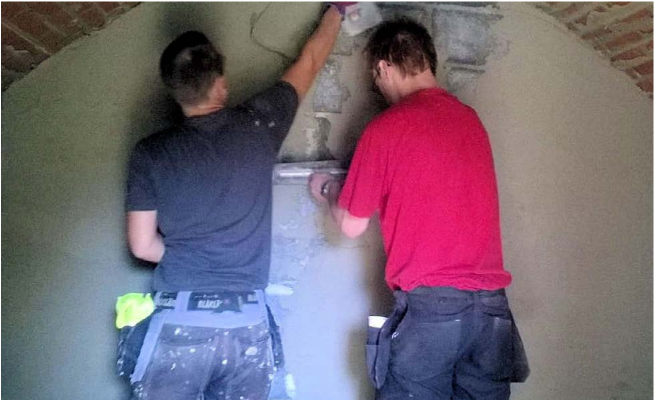
FIGURE 3.2. Plastering a wall takes a lot of practise. These students obviously knew the trade. Photograph by Kirsti Horn.
