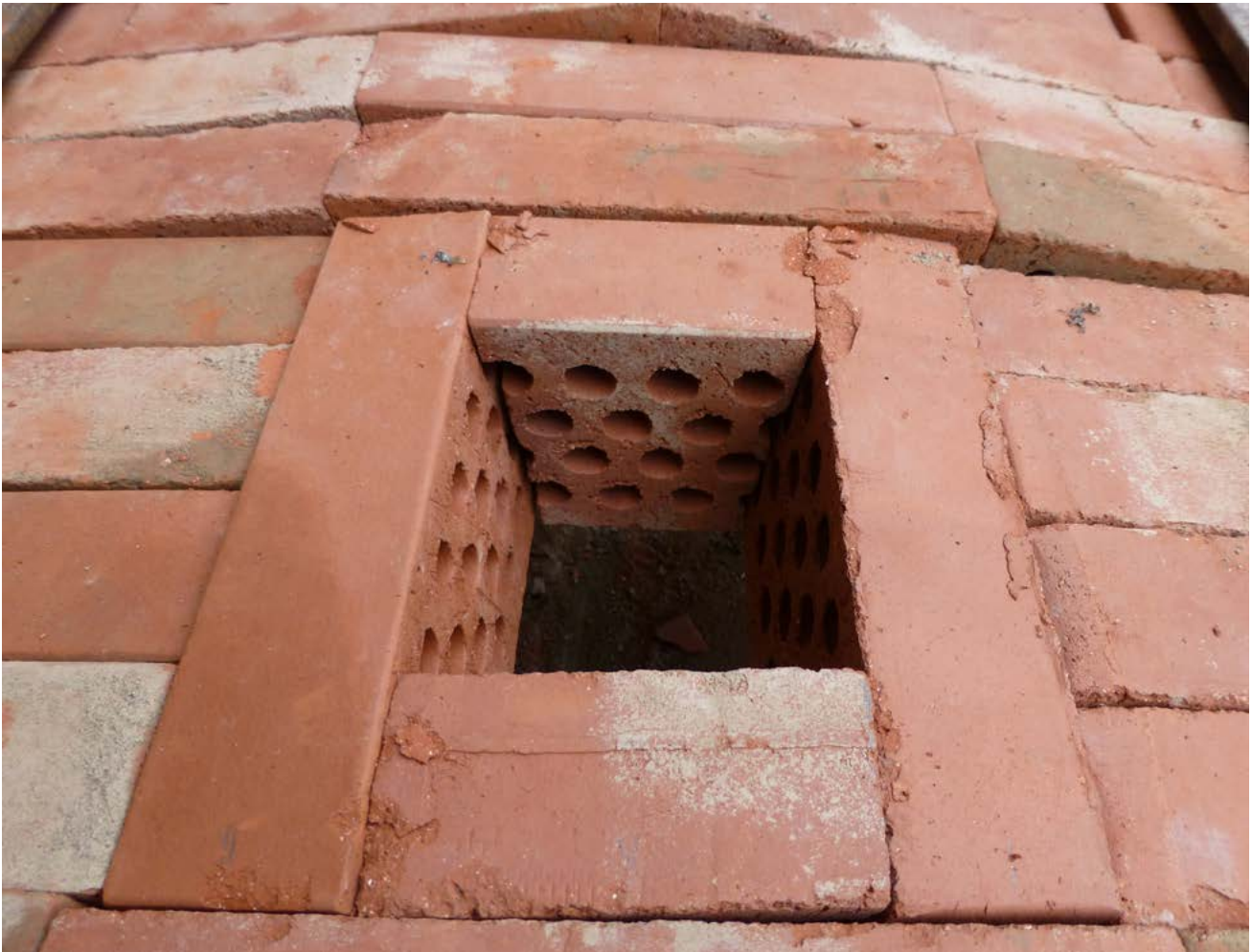
FIGURE 2.24. Note how the two back rows are made with waste pieces from the bricks of the front rows at the ends. Alternating the two types would give a stretcher bond. Photograph by Kirsti Horn.
