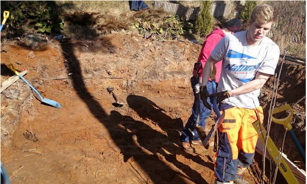
FIGURE 2.2. The surface of the plot is levelled to the depth of the plinths and the drainage pipe. Photograph by Niklas Nyman.
