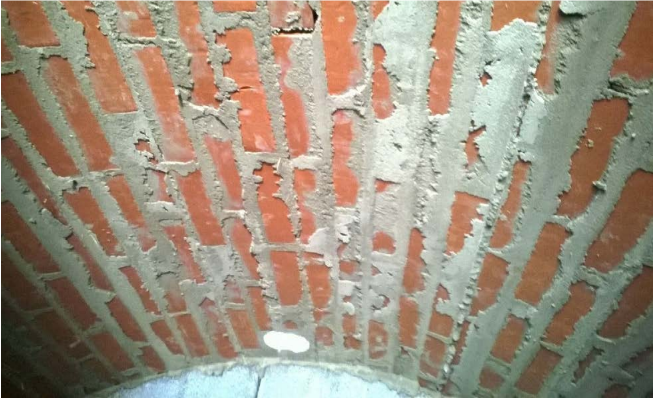
FIGURE 2.19. The completed vault. When the formwork was removed we could see that we had used too much mortar in some places and too little in others. Photograph by Kirsti Horn.
