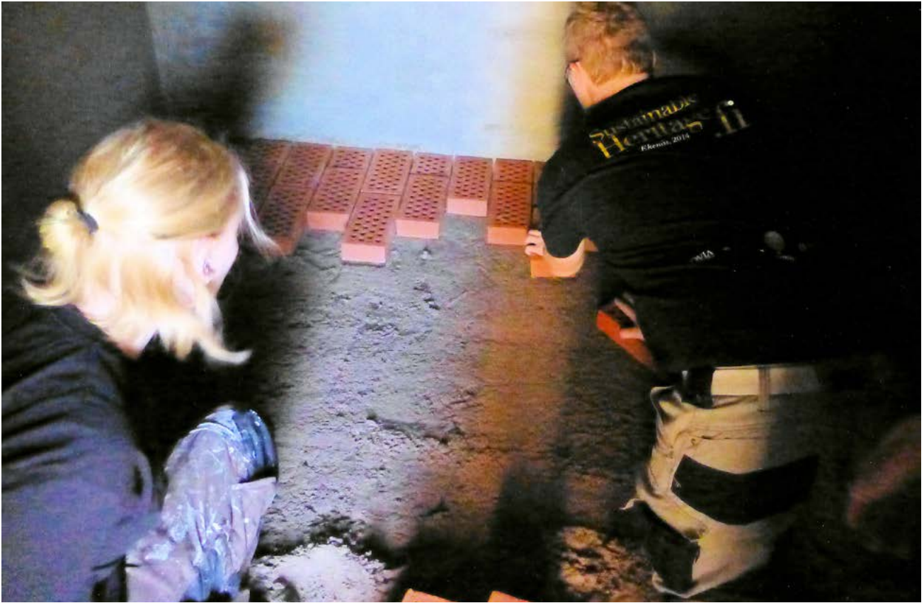
FIGURE 3.6. Air bricks are being laid on the bed of sand. Photograph by Kirsti Horn.
